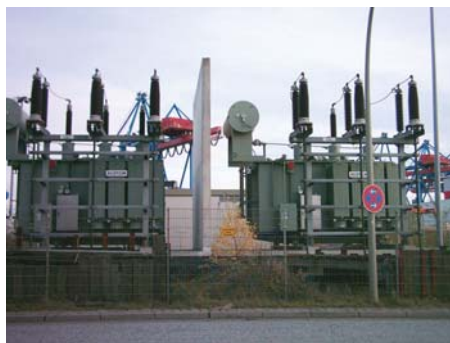
Figure 20.19 Power is distributed over large distances at high voltage to reduce power loss in the transmission lines. The voltages generated at the power plant are stepped up by passive devices called transformers (see Transformers ) to 330,000 volts (or more in some places worldwide). At the point of use, the transformers reduce the voltage transmitted for safe residential and commercial use. (Credit: GeorgHH, Wikimedia Commons)
